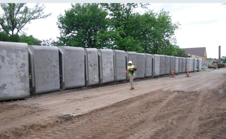
Twenty-four 12' x 8; concrete box culvert sections staged for installation on 4th Ave SE
