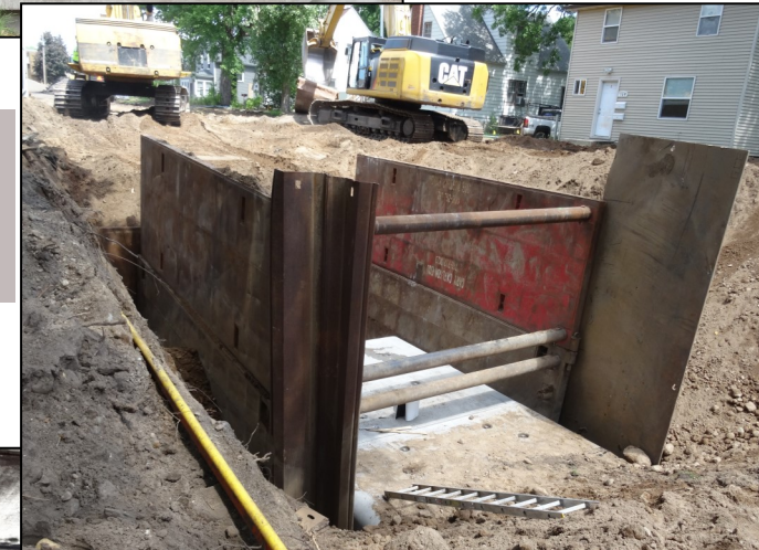
Right: Metal sides used during installation to prevent soil from falling into the structure
