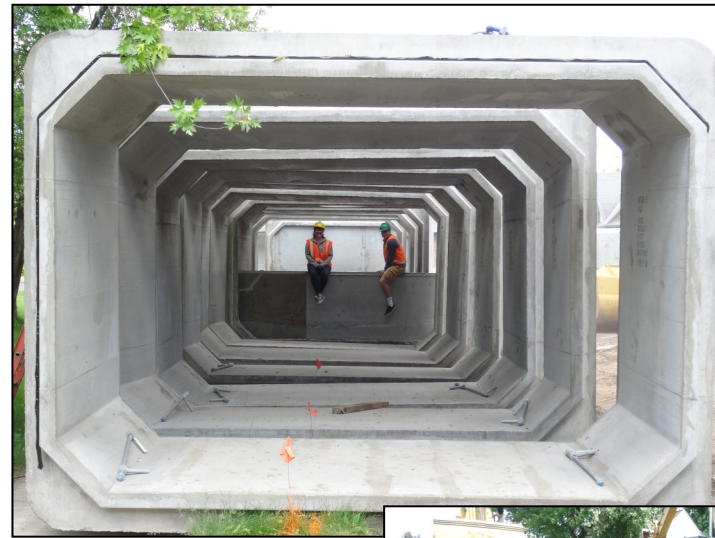
Left: Series of box culverts with weir structure used to settle out solid materials
